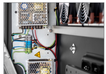
Cabling according to VDE guidelines
